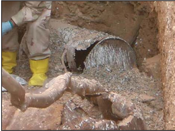
Figure 20. Sloping trenches with exposed drums and debris.
