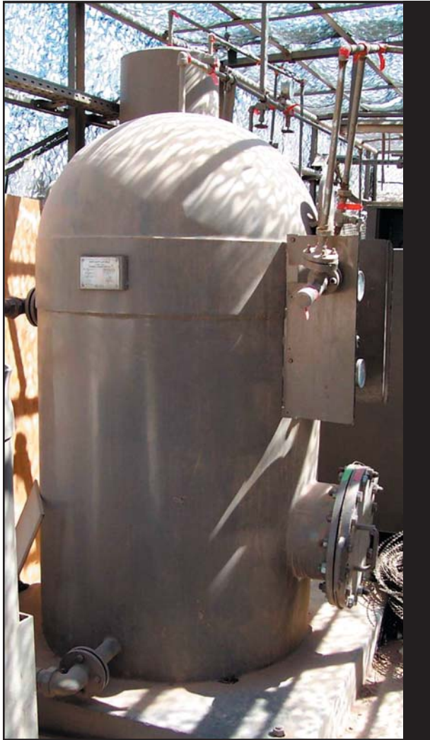
Figure 3 (a). Trailer 1 reactor vessel.
