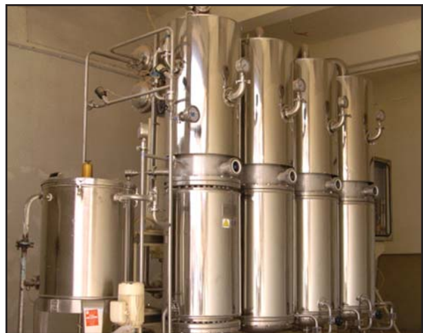
Figure 8. High grade water production plant.
