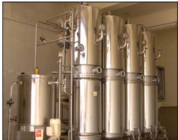
High grade water production plant.
