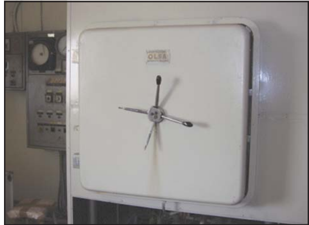
Autoclave with control panel.
