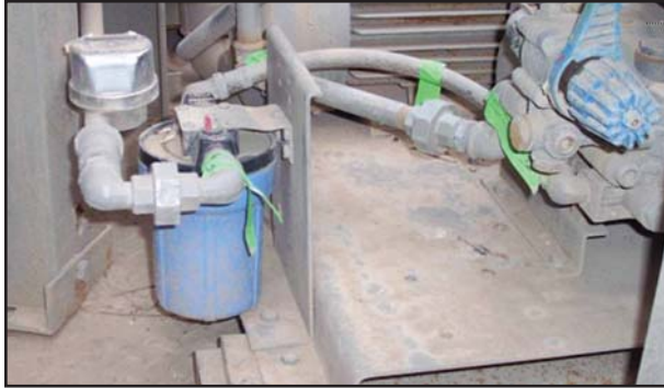
Figure 5. Trailer 1 water filter.
