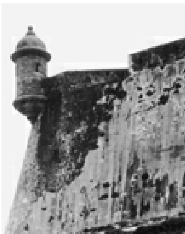
Within the context of Section 106 review, an international team of conservation experts recommended ways to protect existing fabric and slow decay of the defensive walls surrounding the San Juan National Historic Site.
