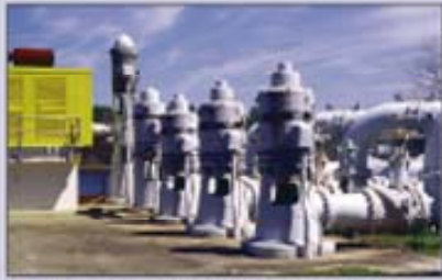
Public supply water intake, Bay County, Florida
