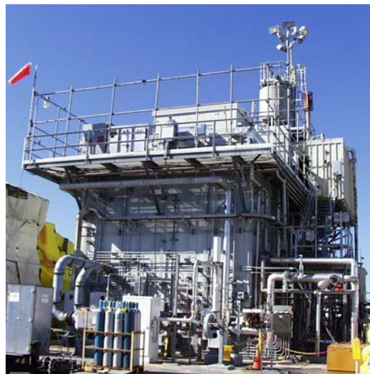
The site’s three evaporator facilities work together to create much needed space within the SRS tank farm system.
