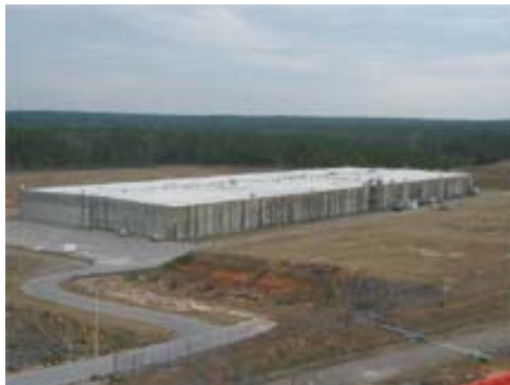
Each Vault 4 cell at the Saltstone Processing Facility is capable of containing about one million gallons of grouted material. All of the decontaminated salt solution received from MCU is expected to be permanently stored within the 10 Vault 4 cells.
