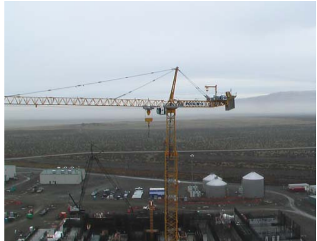
A crane like this one at Hanford was dismantled and shipped to SRS on 22 truck loads to help with the construction of the MOX plant.
