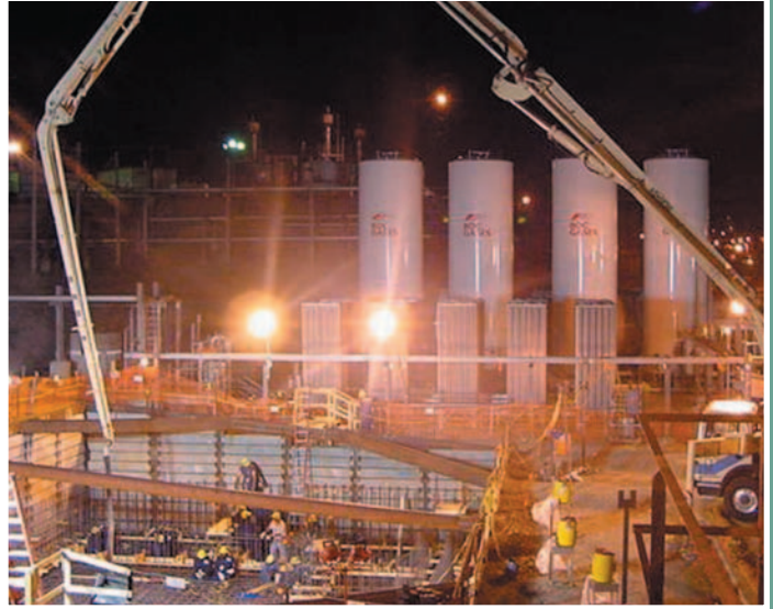
▲ Construction is under way on the Modular Caustic Side Solvent Extraction Unit, which will process some of the salt materials in SRS' waste tanks.
