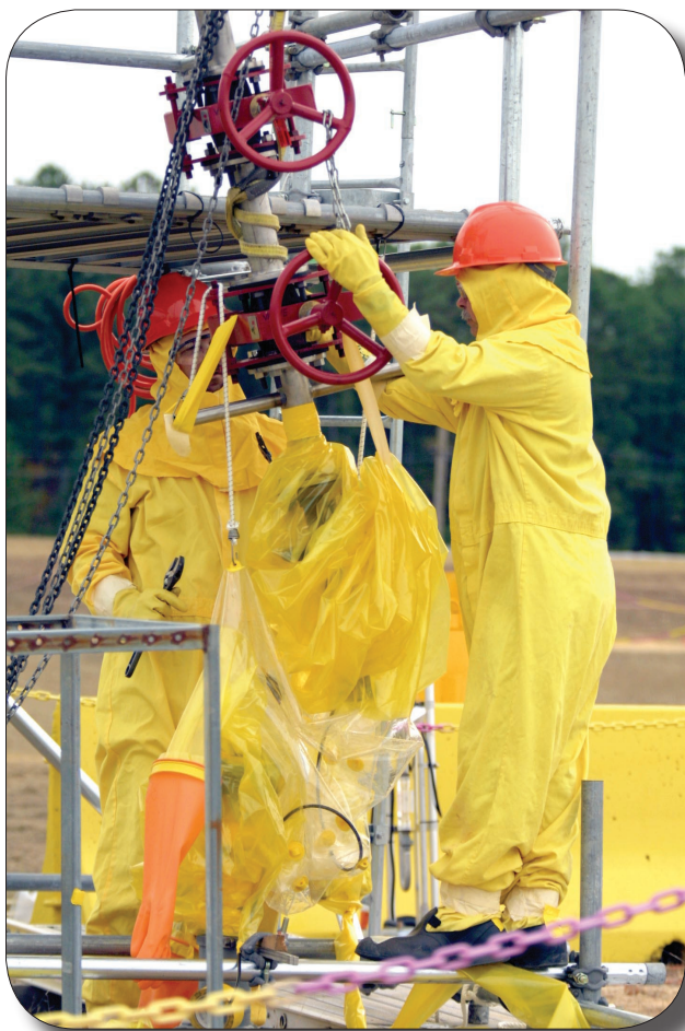
Workers install equipment in preparation for another grout pour at the Old Radioactive Waste Burial Ground solvent tank closure project
