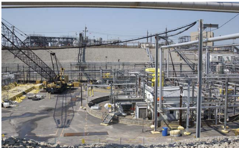
F Area's tank farm contains the first two closed tanks, with two more slated to be closed before the end of 2006.
