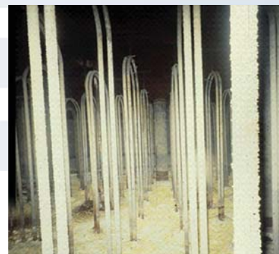
Inside a high-level waste tank.
