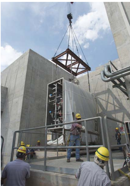
Construction of the Tritium Extraction Facility began in 2000 and is approximately 50 percent complete.
