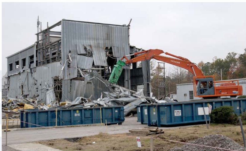
Building 313-M, one of many reactor materials facilities in M Area, is demolished.
