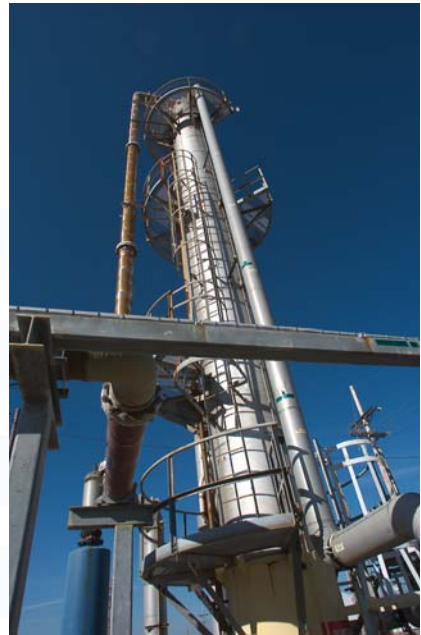
Many millions of pounds of contaminants have been removed from groundwater at SRS by air strippers.
