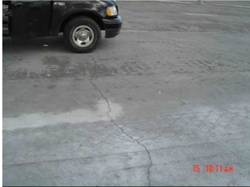
Figure 2-3. Shrinkage cracking in CTB.
