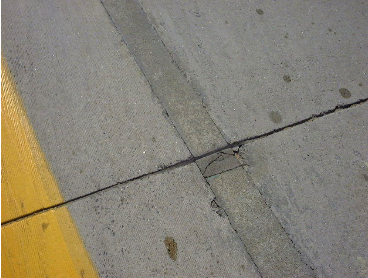
Photo 3 - Joint Spall at Electrical Duct
