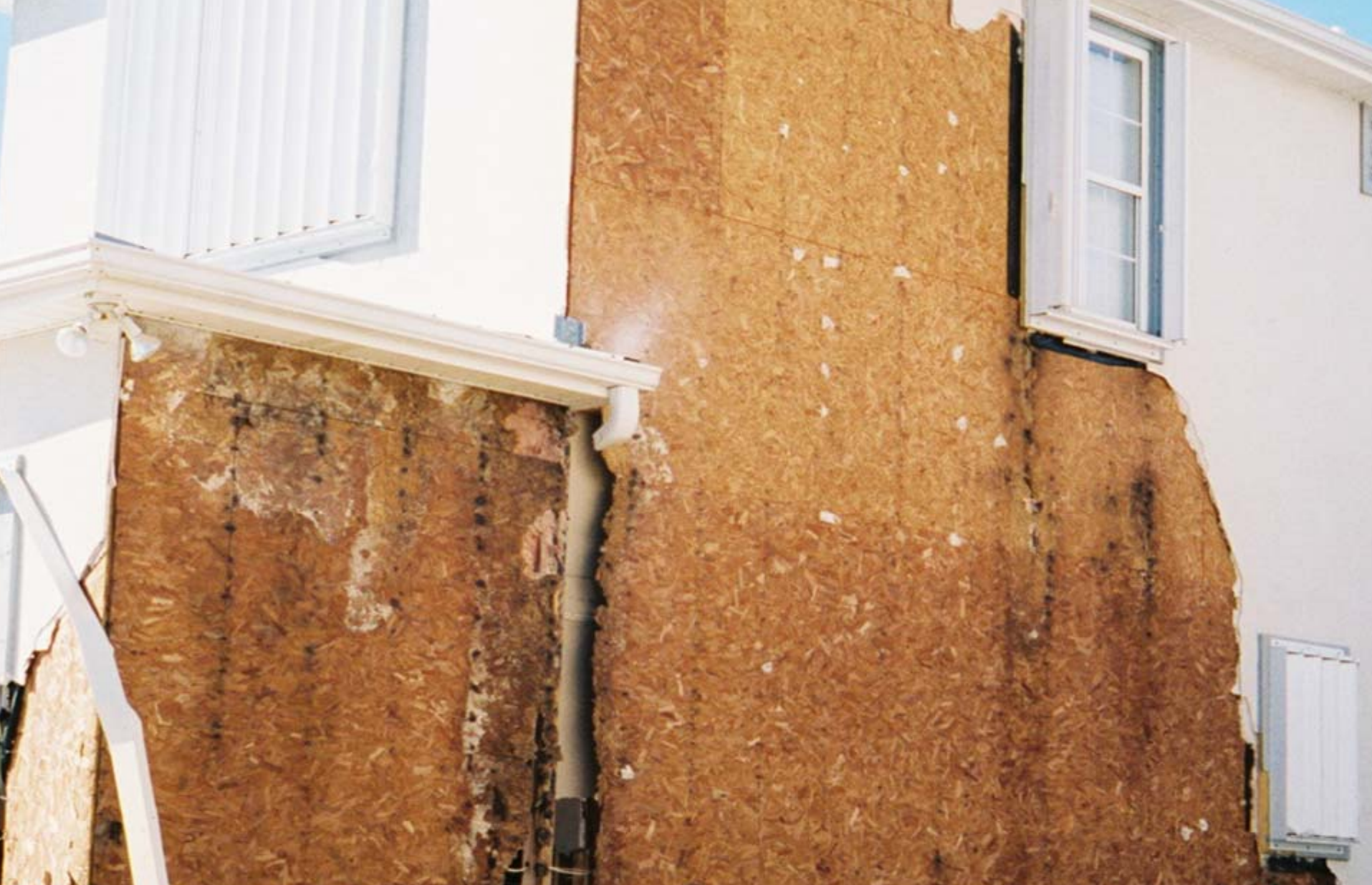
EIFS Failure Navarre Mainland
