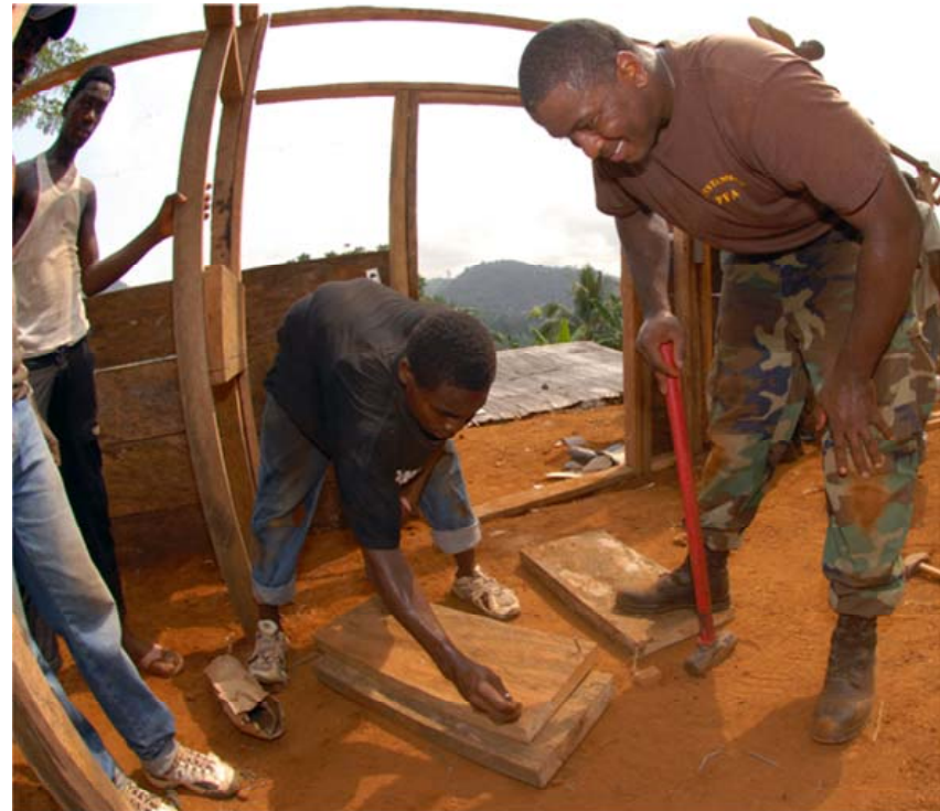
U.S. Navy Utilitiesman 2nd Class Gregory Knight volunteers with members of the Organization of Limbe United Youth Associations to build a doorframe in Limbe, Cameroon, Dec. 11, 2007, as part of the African Partnership Station (APS). APS is a multinational effort to bring the latest training and techniques to maritime professionals in nine West African countries.
