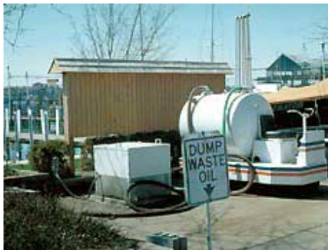
Pump-out stations at marinas such as this one allow boaters to empty their sanitary systems without contaminating the water. Click on image for larger view.
