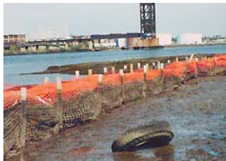
Similar to sediment fences, retaining fences are used to prevent contaminants from entering aquatic environments. Click on image for larger view.
