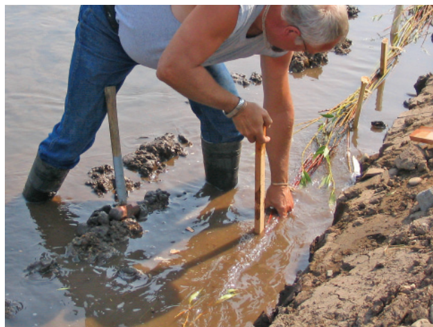
▲ During FY 2005-2006, the Confederated Tribes of the Umatilla Indian Reservation removed 1,400 linear feet of the Fletcher levee and 2,200 cubic yards of associated cobble and rock fill in Camas Creek in the north fork of the John Day River basin in Oregon.
