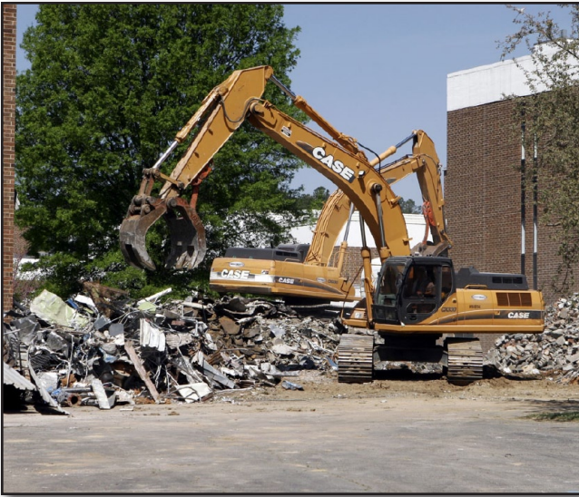
A Case swing excavator can crawl over almost anything with its tank-like tracks and demolish steel-reinforced brick walls with ease. (Photo courtesy of Steve McCaw)
