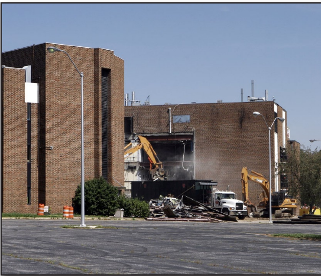
Construction dust rises as the excavator loads debris into dump trucks for removal. (Photo courtesy of Steve McCaw)
