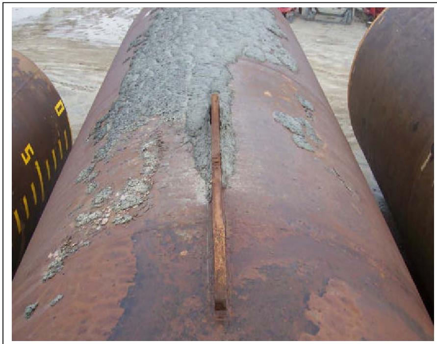
Figure 18: Shows the Damaged Padeye on the Suction Piles. The padeye angle was about 45° at the time of failure.
