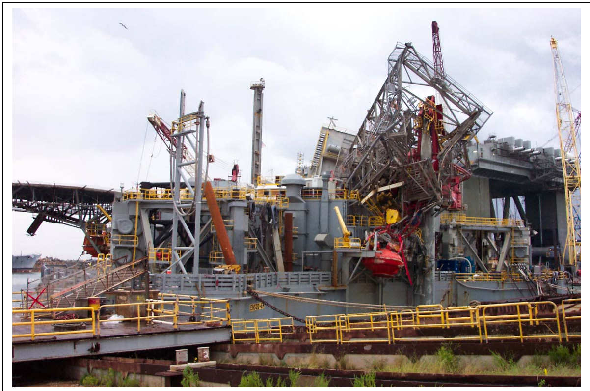
Figure 33: Photo showing the derrick collapsed.
