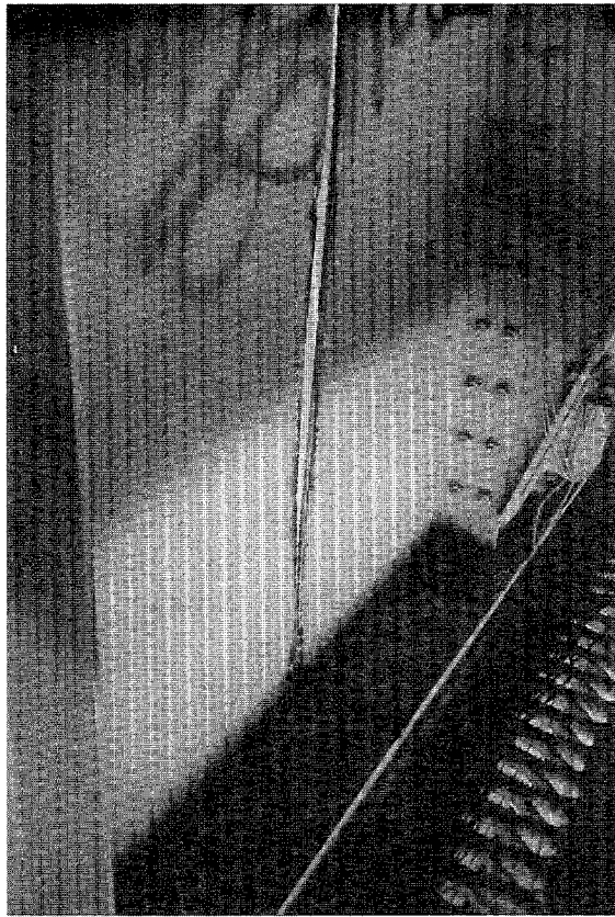
Fig. 19. Third stage of damage: six-foot cut in the web and cuts through half the bottom flange on either side of the web.
