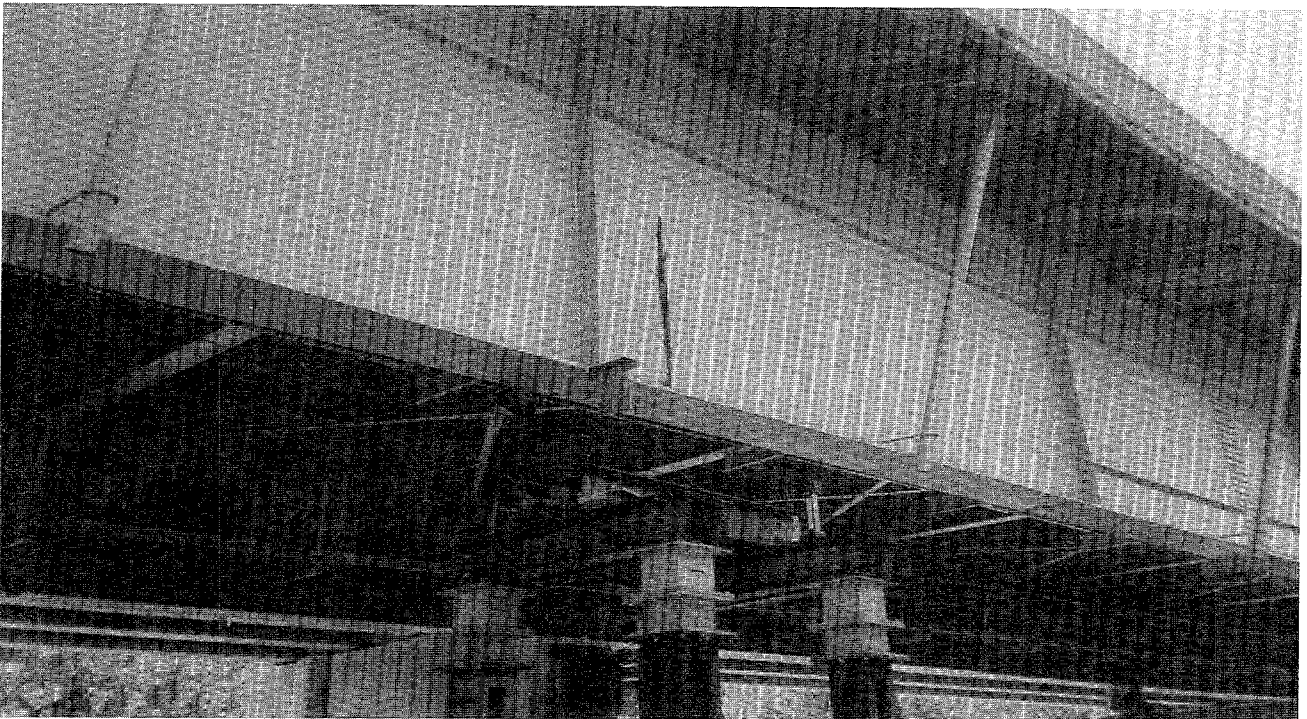
Fig. 18. Second stage of damage: six-foot cut from the center of the web to the bottom flange.
