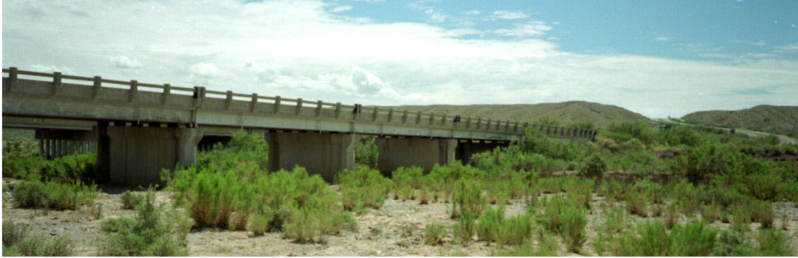
Figure 3. The measured fundamental frequency of this Alamosa Canyon Bridge in New Mexico varied approximately 5% during a 24-hour test period. This variation emphasizes the importance of data normalization. (Sohn et al. 2001)
