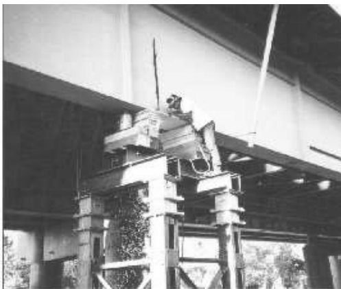
(a) Introduction of damage in one of the bridge girders by electric saw cutting.
