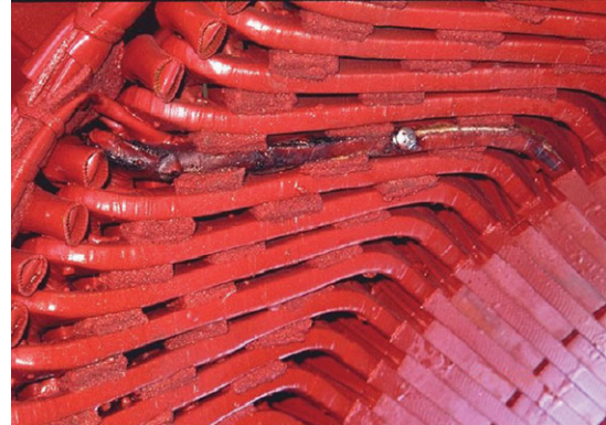
Figure B8 Staged stator insulation fault.
