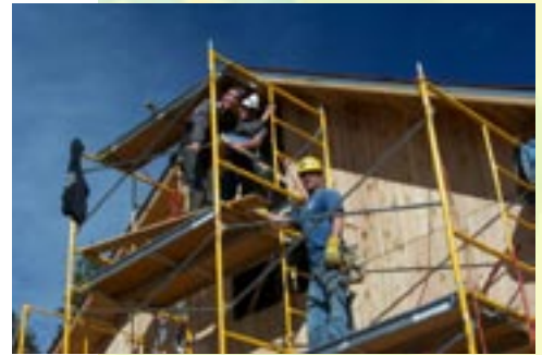
Recreation Solutions Archaeology and Historic Structures Branch lead (r) and volunteers installing new siding during restoration of the Aldo Leopold House on the Carson National Forest in New Mexico.
