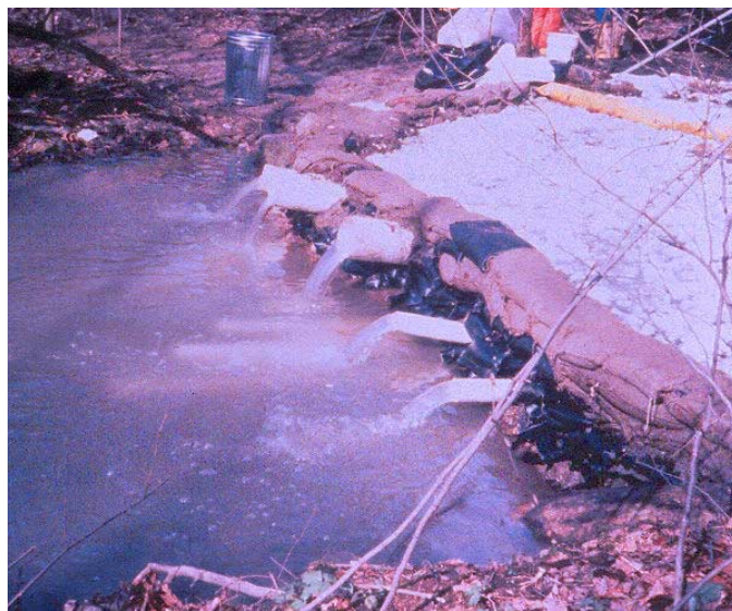
Figure 4-22. Sandbag underflow dam.
