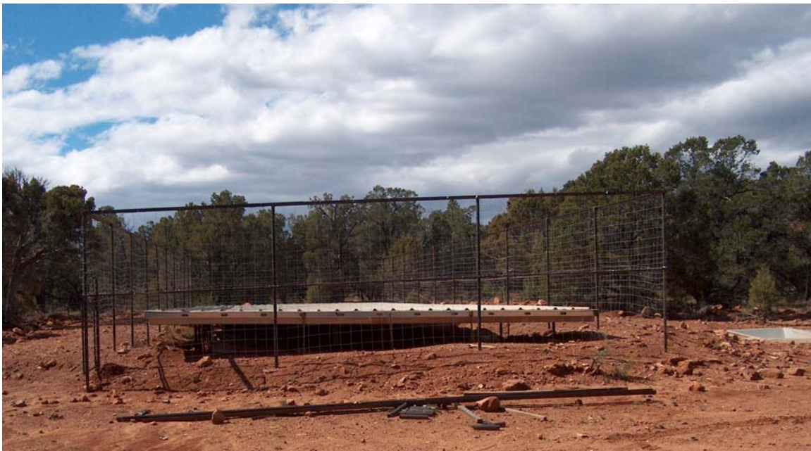
Figure 2. Reconstructed Wildlife Water Catchment: Underground Water Storage Tanks, Collection Apron, Field Fence, and Drinker (to the right). Site area still needs to be graded and seeded.
