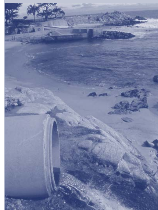
A stormdrain outfall pipe discharges into the ocean near Lover's Point in Pacific Grove.
