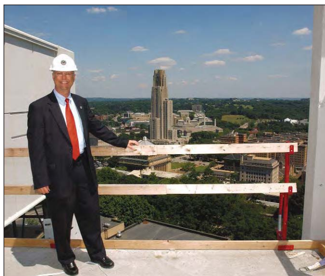
Mr. Moreland stands atop of the highest point of the nine-story parking garage being constructed at VA Pittsburgh Healthcare System.
