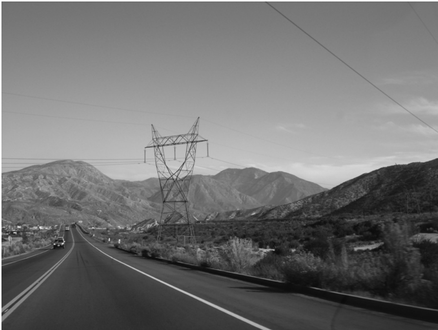
Utility corridor, Cajon Pass
