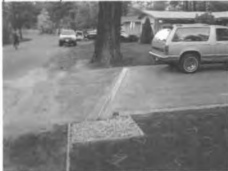
Slotted drain and drywell to infiltrate driveway runoff.
