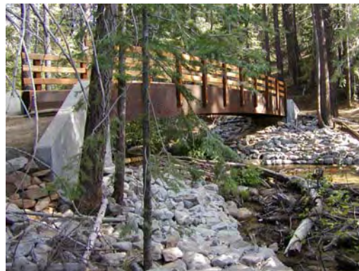
After: Beaver Creek Trail Bridge with larger flow area, improved soil erosion measures, and safe structure.
