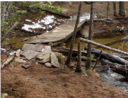
Before: Beaver Creek Trail Bridge with inadequate soil erosion measures and failing structure.
