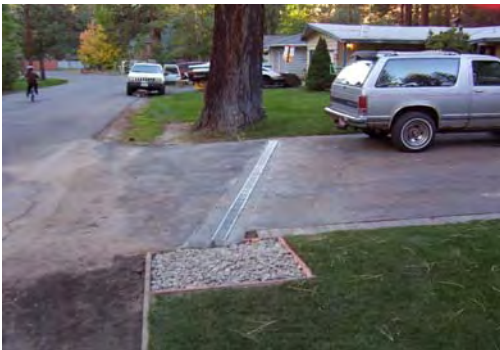
Slotted drain and drywell to infiltrate driveway runoff on a residential property.
