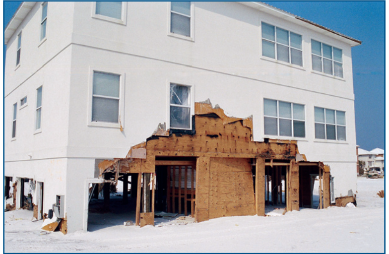
Siding on the non-breakaway portions of this elevated building was extended over breakaway enclosure walls and was damaged when breakaway walls failed under flood forces.
