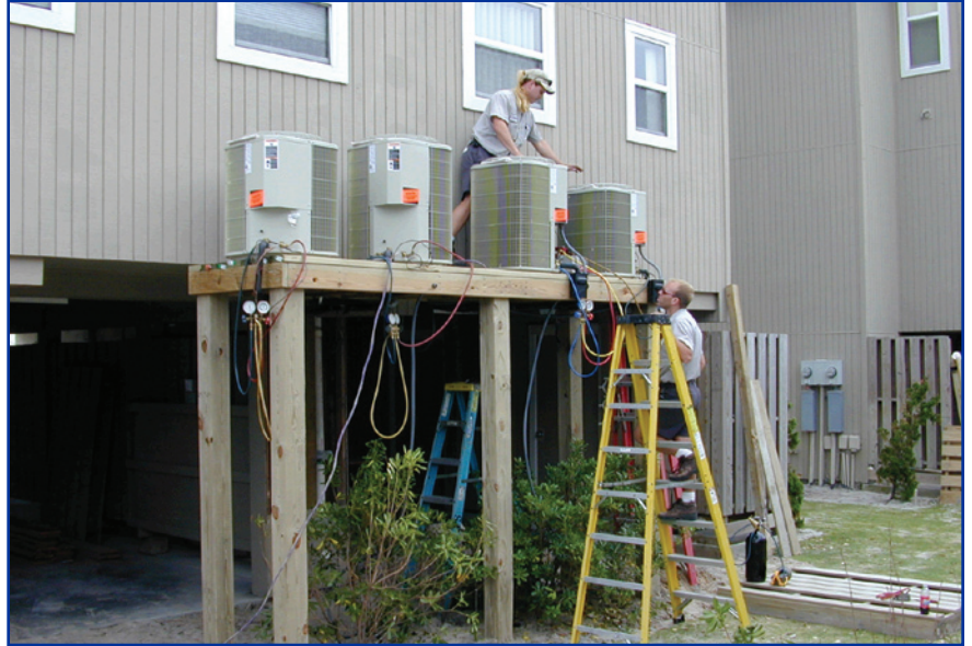
Elevated air conditioning compressors.
