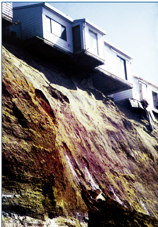
House undermined by bluff erosion. Photograph by Lesley Ewing. Courtesy of California Coastal Commission.
