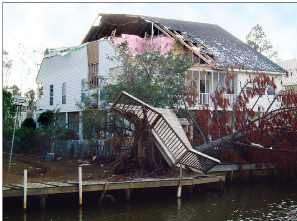
Figure 1-1. Wind damage to roof structure and gable end wall from Hurricane Katrina (2005) (Pass Christian, Mississippi)
