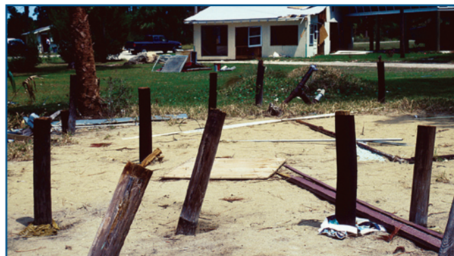
Insufficient pile embedment and failure of connections at tops of piles allowed elevated building to be floated off its foundation.
