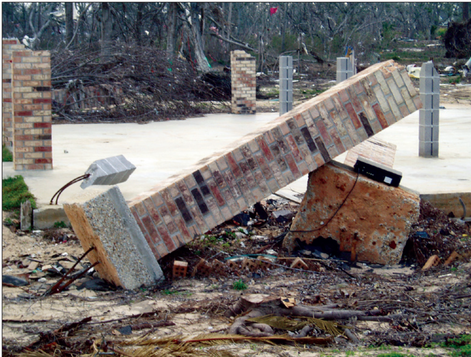
Figure 2-7. Performance comparison of pier foundations. Piers on discrete footings (foreground) failed by rotating and overturning while piers on more substantial footings (in this case a concrete mat) survived (Pass Christian, Mississippi)
