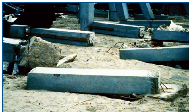
Pier (column) failures: footings undermined and columns separated from footings.
