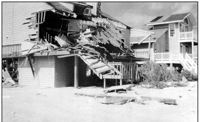
Figure 2. Well-sited building that still sustained damage.
