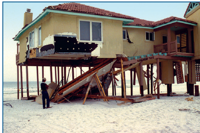
Pile failures led to collapse of floor of elevated building.
