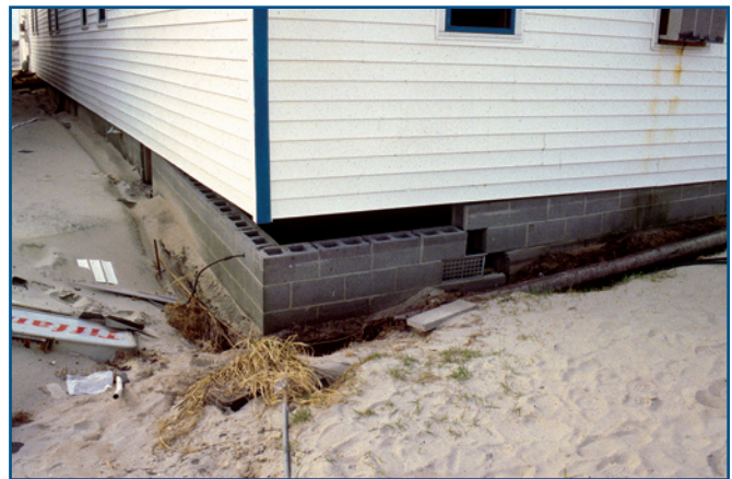
Failure of crawlspace foundation undermined by scour.
