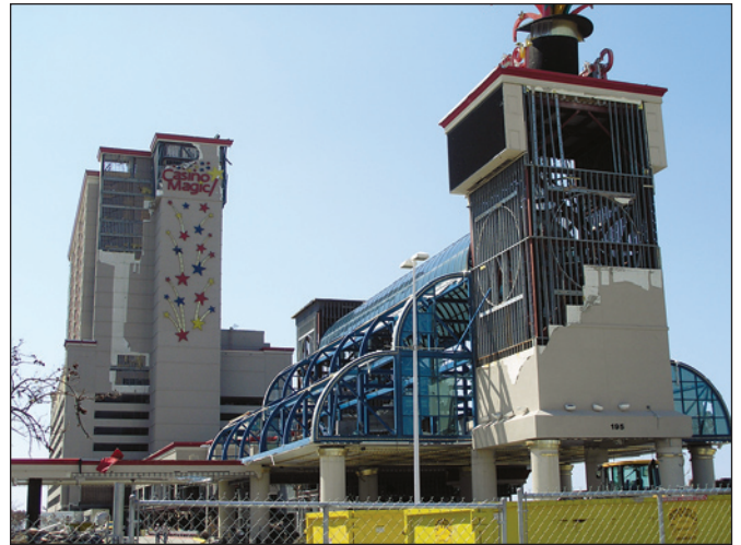
Figure 2-18. Multi-story building showing severe EIFS damage. In some areas, the gypsum board on the interior side of the studs was also blown away (Biloxi, Mississippi).
