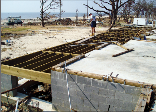
Figure 2-7. Stem wall foundation survived intact, but waves and surge above the floor destroyed the house, sweeping it off the foundation (Waveland, Mississippi).
