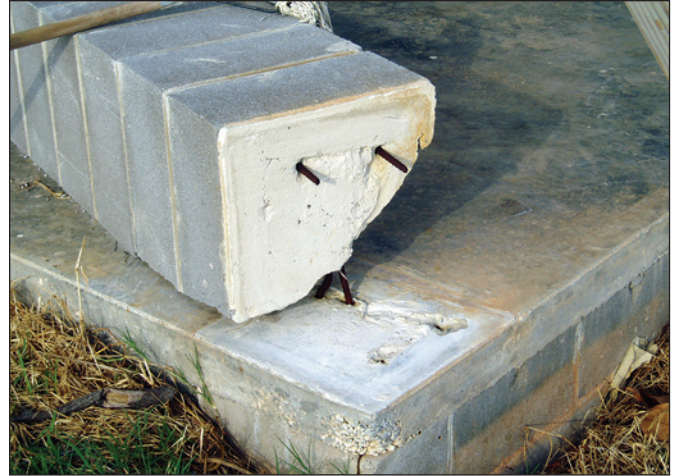
Figure 2-4. Pier connection failure (Belle Fontaine Point, Jackson County, Mississippi)
