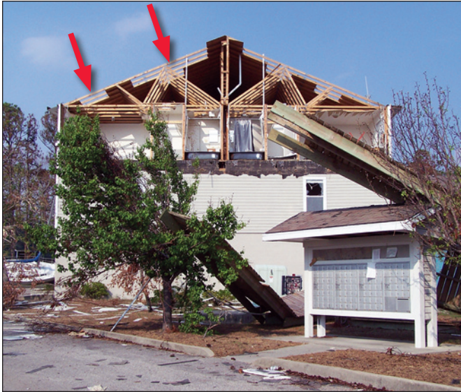
Figure 2-12. Failure of the gable end wall of this apartment building led to pressurization of the attic and the release of sheets of plywood sheathing. Note the plywood roof sheathing “unzipped” by wind pressures (arrows), (Ocean Springs, Mississippi).
