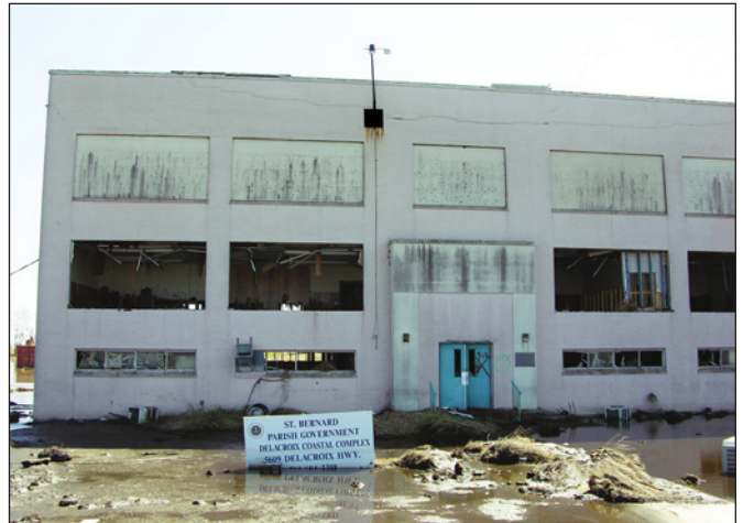
Figure 3-6. Storm surge damage to the St. Bernard Parish Coastal Government Complex (Delacroix, Louisiana)
