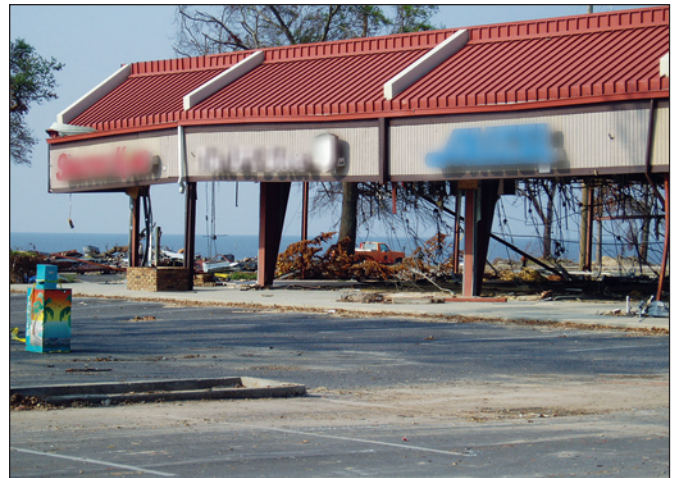
Figure 2-8. Steel frame strip mall construction with exterior wave damage (Gulfport, Mississippi)
