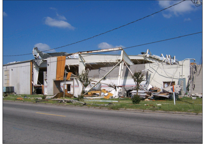
Figure 2-16. Pre-engineered metal building failure (Gulfport, Mississippi)
