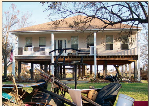
This photo was taken post-Katrina, illustrating the survival of this elevated building.
