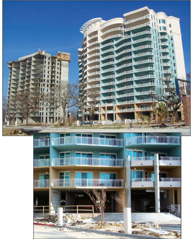
Figure 2-9. High-rise buildings along Beach Boulevard received non-structural flood damage to the lower floor, and no apparent flood or wind damage to higher residential floors (Gulfport, Mississippi)
