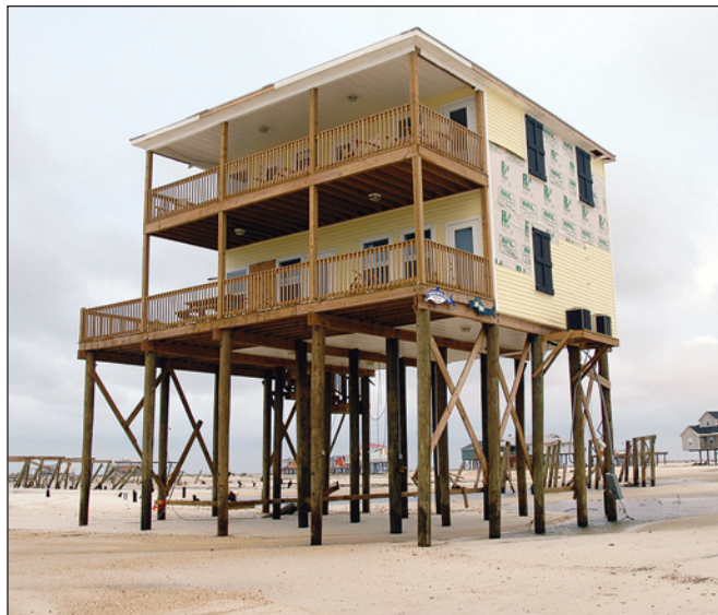
Figure 2-1. Successful example of well-elevated and embedded pile foundation following Katrina. Note adjacent building failures where foundations were not high enough or where pile embedment was insufficient (Dauphin Island, Alabama).
