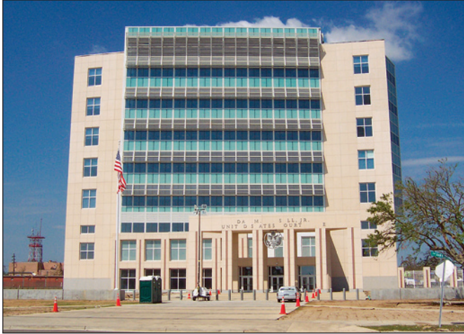
Figure 2-15. Reinforced concrete/steel frame building that performed well structurally, but did have some building envelope damage and roof mounted HVAC equipment damage (Gulfport, Mississippi)
