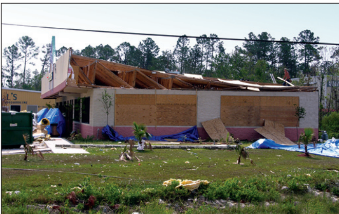
Figure 2-13. Failure in a wood frame commercial building. Trusses lost roof sheathing, allowing trusses to tip over (Ocean Springs, Mississippi).
