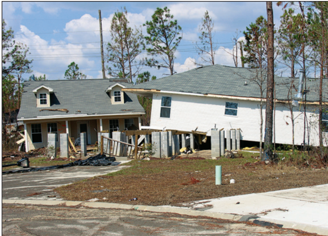
Figure 2-5. Buildings floated off of pier foundations (Pass Christian, Mississippi)
