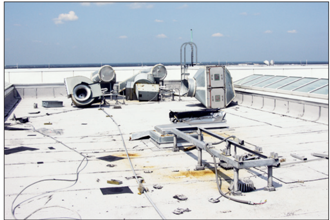
Figure 2-21. The equipment on this new Federal courthouse blew away because it was resting on vibration isolators that provided lateral resistance, but no uplift resistance. Two large openings through the roof were left after the ductwork blew away (temporary covers had been placed over the openings).
