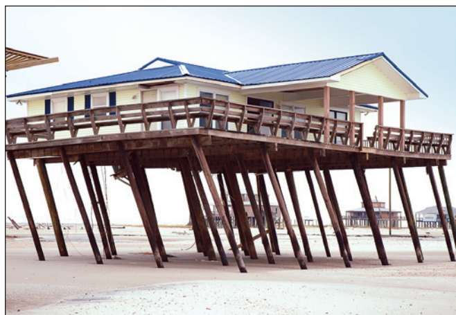
Figure 2-2. House that nearly failed due to insufficient pile embedment (Dauphin Island, Alabama)
