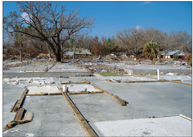
Figure 2-6. Waves, surge, and floating debris destroyed many single-family homes on slab foundations. Note the debris from houses that washed landward into other buildings (Biloxi, Mississippi).
