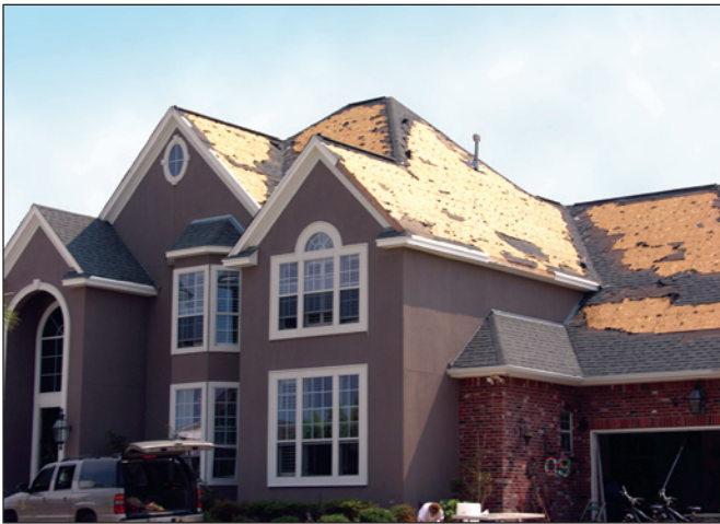
Figure 2-17. Extensive loss of roof covering and underlayment (Slidell, Mississippi)
