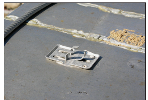
Figure 3. During high winds, the conductor deformed the prongs and pulled away from this conductor connector.
