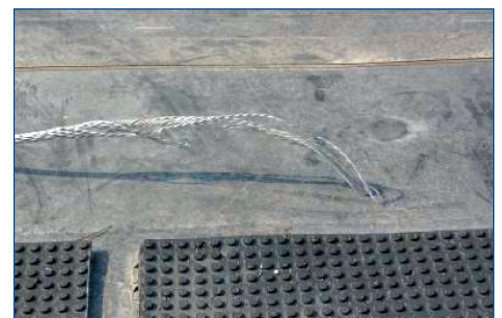
Figure 2. View of an abraded end of a conductor that became disconnected.
