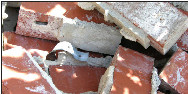
Figure 3. This tie remained embedded in the mortar joint while the smooth-shank nail pulled from the stud.
