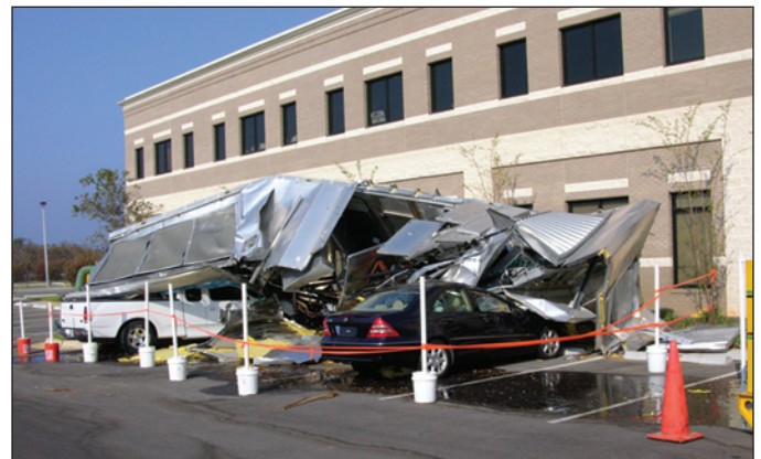
Figure 2. This 30' x 10' x 8' 18,000-pound HVAC unit was attached to its curb with 16 straps (one screw per strap). Although the wind speeds were estimated to be only 85 to 95 miles per hour (3-second peak gust), it blew off the building.
