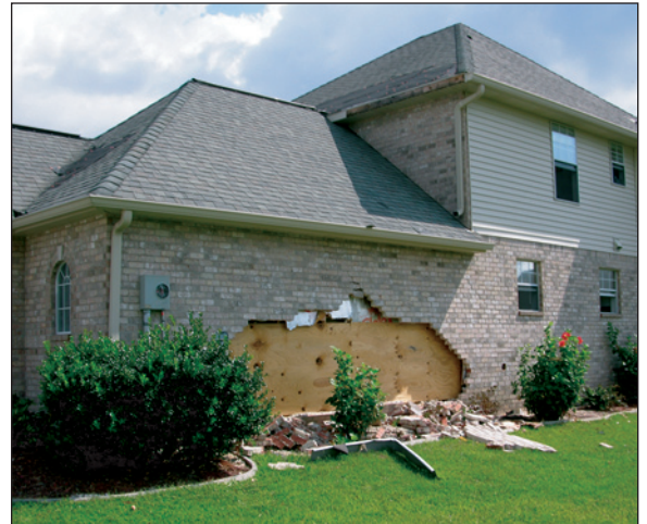
Figure 1. Failed brick veneer. Plastic foam wall sheathing was installed over the wood studs (plywood was temporarily installed after the brick failure).
