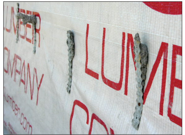
Figure 4. These four ties were never embedded into the mortar joint.
