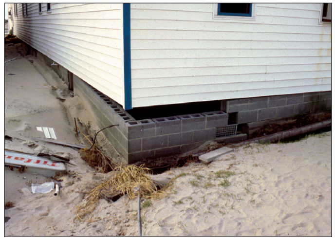
Figure 4. Failure of A Zone type foundation in coastal area, not subject to V Zone conditions (Hurricane Fran).
