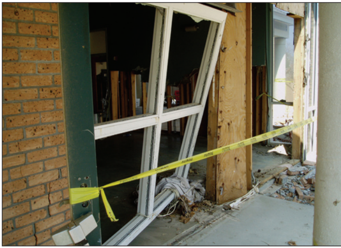
Figure 3. Failure of wood-frame wall, brick veneer, and windows as a result of 4 feet of stillwater flooding and small waves (Hurricane Katrina).
