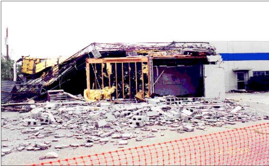
FIGURE 5-27: Additional structural damage caused by breach of envelope in Wichita, Kansas.
