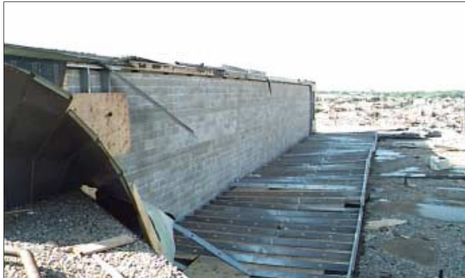
FIGURE 5-24: This metal-clad wall covering collapsed and in other areas it was blown completely away.
