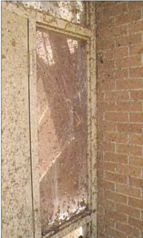
FIGURE 5-25: The corner of a table penetrated this laminated glass, but the glass remained in its frame. This school suffered major damage from inflow winds of a violent tornado in Moore, Oklahoma.
