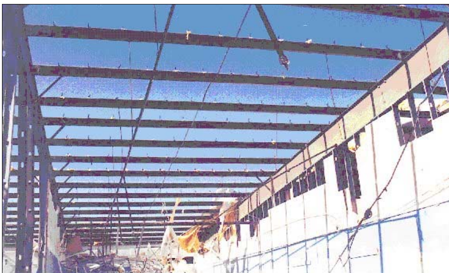
FIGURE 5-5: Metal roof deck of regional outlet mall, Stroud, Oklahoma, blown off when hit by moderate tornado vortex.
