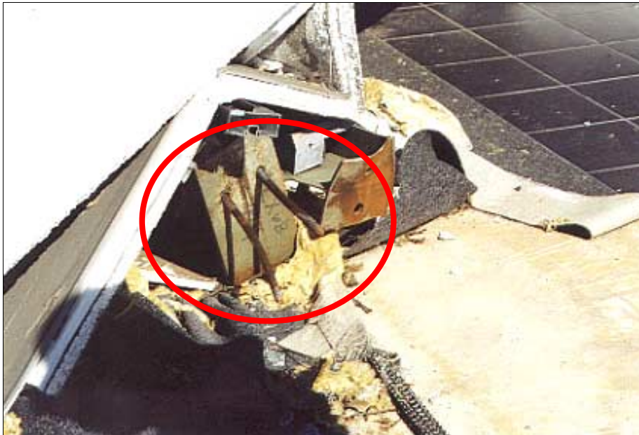
FIGURE 5-8: Column anchors that withdrew from concrete foundation at the regional outlet mall in Stroud, Oklahoma, hit by moderate tornado vortex.
