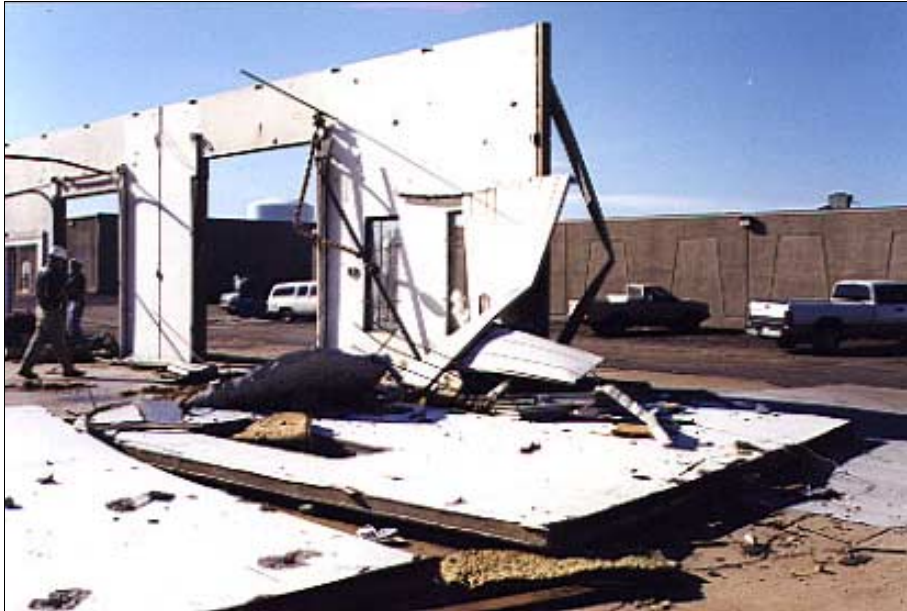
FIGURE 5-2: Tilt-up precast concrete walls at a storage building located outside Del City, Oklahoma. After the roof joists separated from the walls, this end wall became unable to withstand suction forces and failed.
