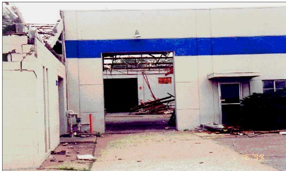
FIGURE 5-19: The tilt-up precast concrete walls in this building did not fail when the roof system failed. Note: many roof joists are still in place. Building was located in Wichita, KS and was hit by moderate tornado vortex.
