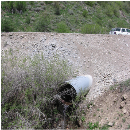
Pre-project Georgetown Road affects aquatic habitat by undersized and impassable culverts and encroachment upon the stream and its riparian area.
