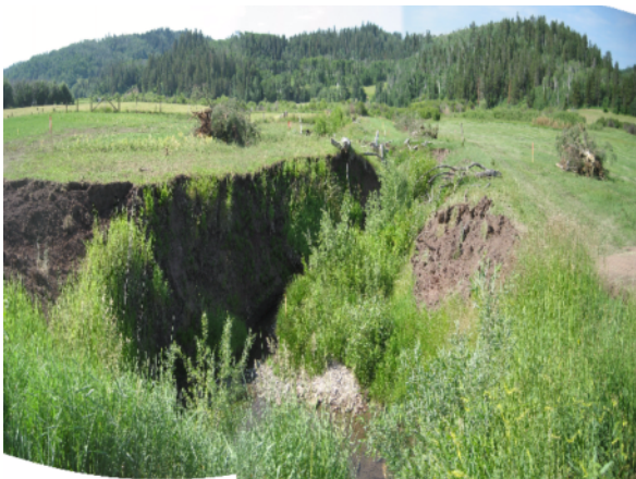
Prior to project implementation, the under-sized culvert at the county road crossing had caused this eroded gully downstream.
