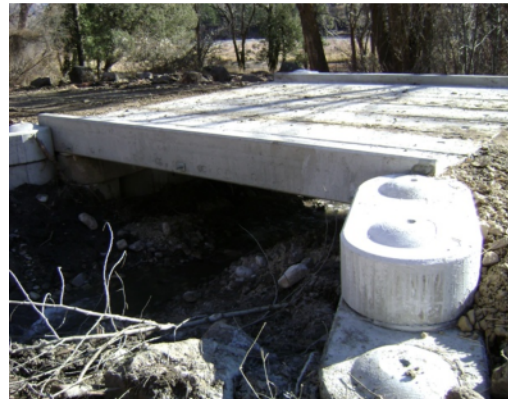
Aquatic organism passage and natural hydrology were restored at the South Fork Snake Road crossing of Wolverine Creek
