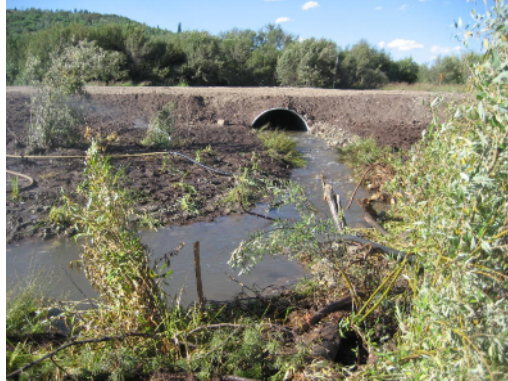
New bottomless arch at county road crossing accommodates upstream fish passage and high flows
