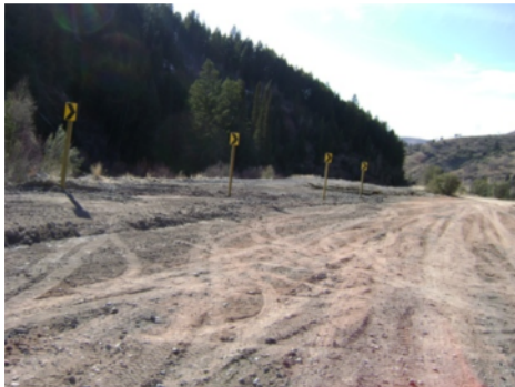
The new Georgetown Road (on the right) veers away from Georgetown Creek and the old road which closely paralleled the stream. The arrows direct users to the new segment road.
