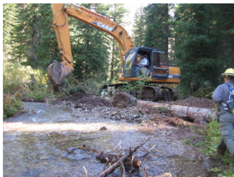
An excavator returns Mail Cabin Creek to its channel from an old road, decreasing erosion and sedimentation.
