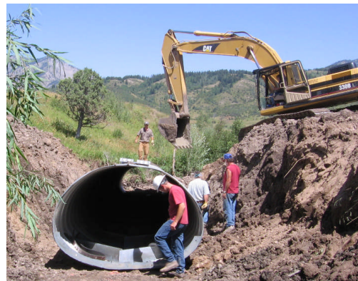
A fish passage culvert is installed under McCoy Creek Road to restore fish passage at Burns Creek, near Palisades Reservoir.
