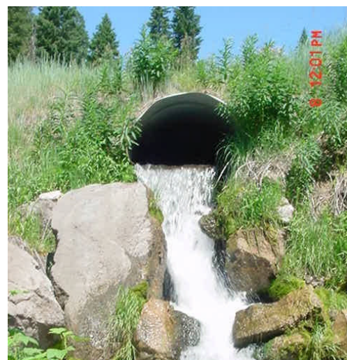
A fish barrier culvert inventoried on Deep Creek in the Soda Springs Ranger District.
