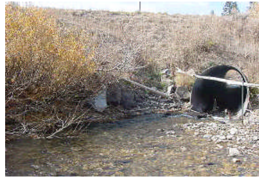
Targhee Creek Culvert under Highway 20 in 2004, before replacement. The culvert was a barrier to upstream-migrating Yellowstone cutthroat trout.
