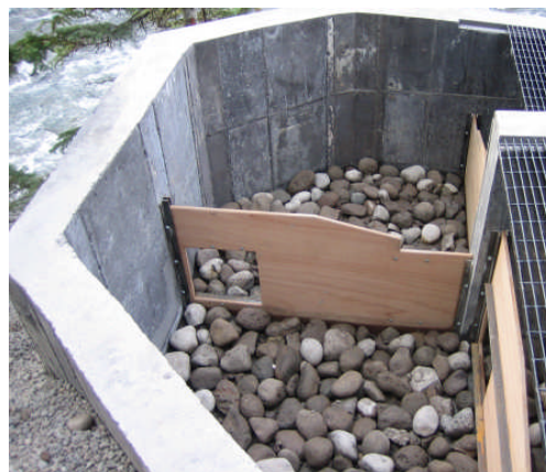
The fish ladder around the Buffalo River Dam was constructed during the summer and fall of 2005 as a result of the relicensing period.
