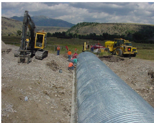
A large, bottomless culvert is placed under Highway 26 by the Idaho Department of Transportation.
