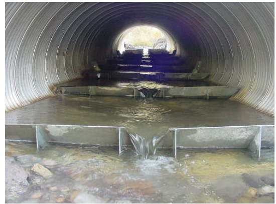
In August 2005, the Trout Creek Fish Passage Culvert was placed under the McCoy Ck Road.
