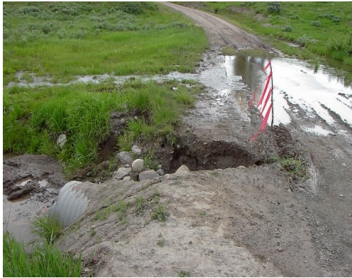
Before the project, the small culvert at Clear Creek would plug and road run-off would erode the fill, delivering sediment to the stream.
