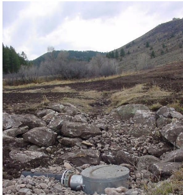
A self-cleaning, fish-screened irrigation pump inlet was placed on the bottom of the new Garden Creek stream channel, within the old pond bed location.
