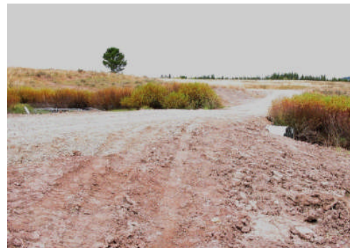
The project included the placement of a larger culvert, and improvement of road drainage.
