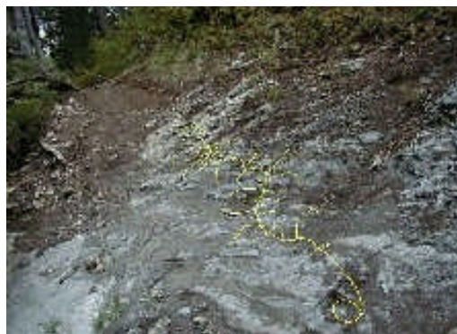
Explosives were used to improve a segment of Burns Creek Trail prior to eliminating illegal riparian trail development in lower Burns Creek.
