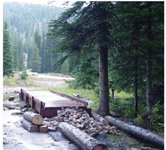
A trail bridge was constructed over Emigration Creek to decrease trail-related sediment delivery to the stream.
