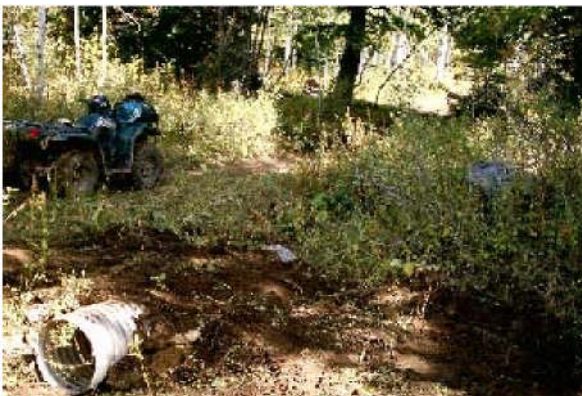
Drainage of the Maple and Sugar Creek trails were improved to decrease sediment delivery to the streams. Here, a culvert was installed under Sugar Creek Trail.
