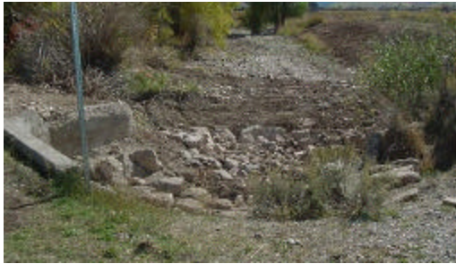
The project removed the concrete sill and added stream roughness to restore upstream fish passage.
