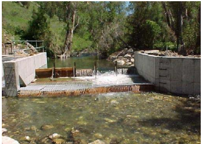
Burns Creek fish weir, constructed in 2000 with USDA Forest Service and other partners' funds.
