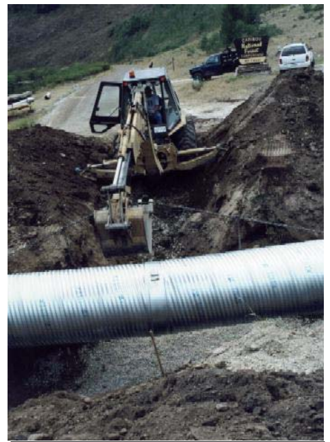
A fish passage culvert is placed at Mill Creek, a tributary to the Blackfoot River.
