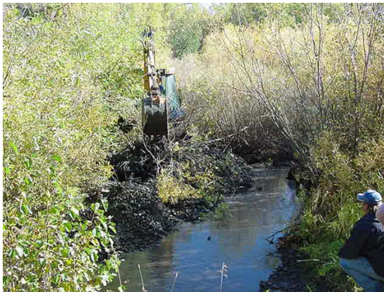
An excavator returns Horseshoe Creek back to its channel after it was captured by a road due to the failure of a culvert on Teton Basin Ranger District.
