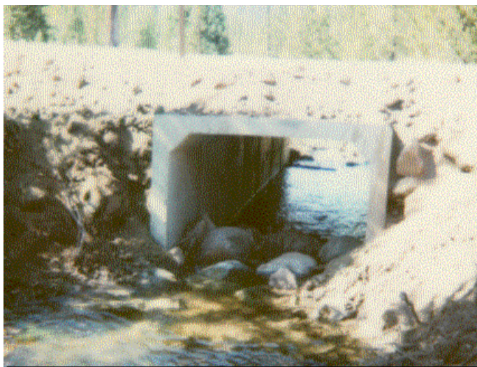
Tygee fish passage conduit after placement. The floor of the concrete conduit simulates a natural stream bottom by retaining some bedload. The conduit grade and elevation is the same as Tygee Creek.
