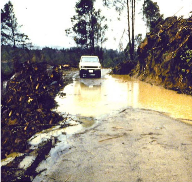
North Fork Caspar Cr., plugged culvert Rd 5
