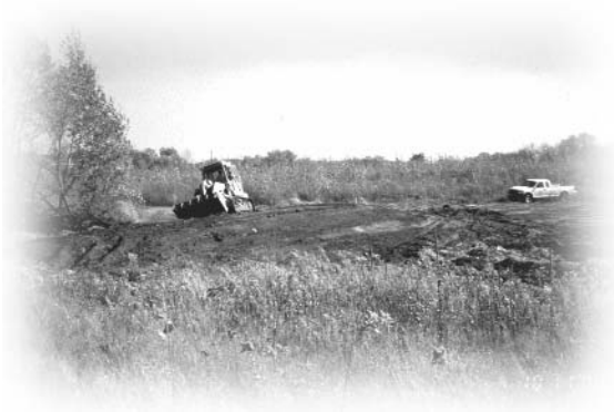
October 2000, dike construction to restore a wetland on the Korf property near Rush Lake, Minnesota.
