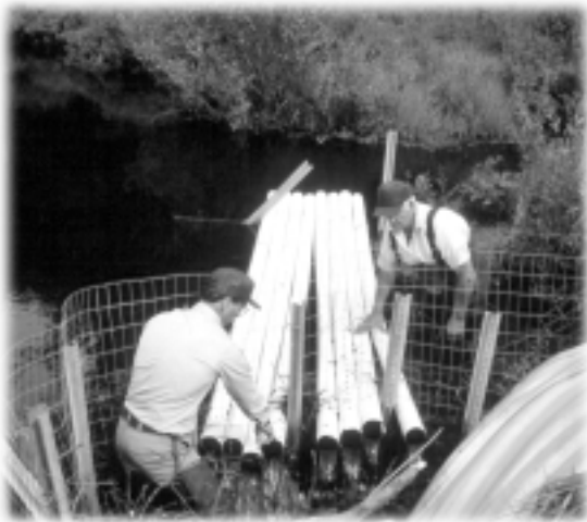
Partners staff in Maine install a beaver exclosure fence and pipes to maintain water levels through a culvert.
