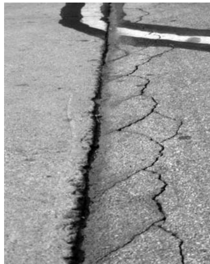
◀ Edge cracking in asphalt along concrete slab.
