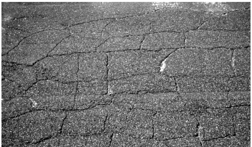
▶ Small blocks with open cracks.
