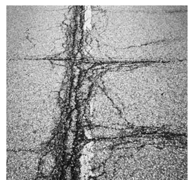
▲ Pavement ravel and erodes along open cracks causing deterioration.
