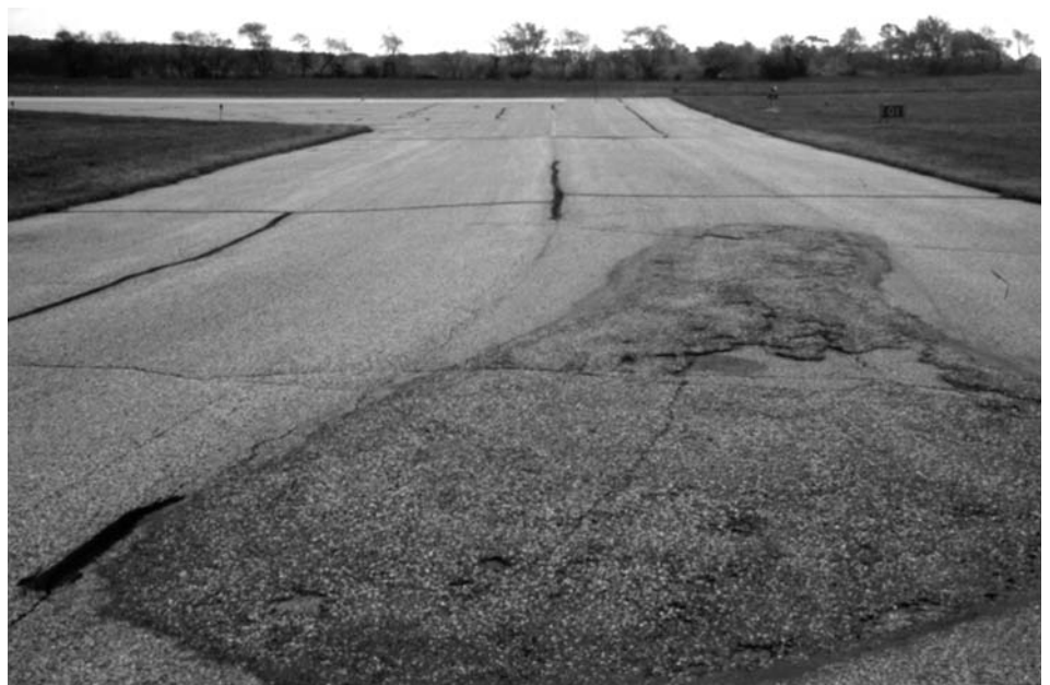
▶ Patch in poor condition.
