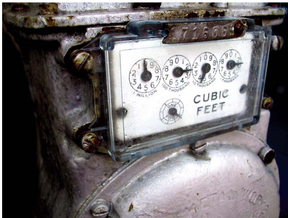
Old equipment poses new problem. Old gas regulators that contain mercury can present a potential health hazard to residents if care is not taken when they are replaced.
