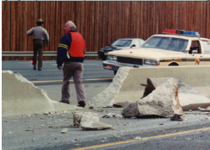
Figure 1-5: Infrastructure damage can occur that requires a timely response.
