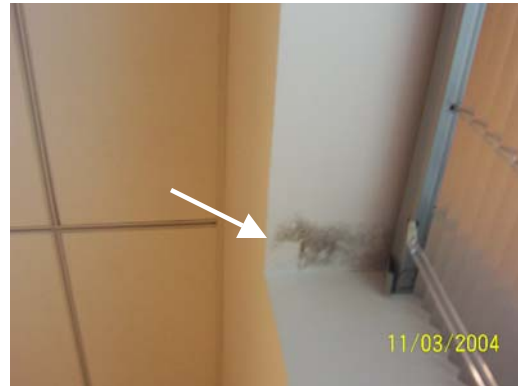
Figure 2. Visible mold on interior drywall at window header in Station 21 office.
