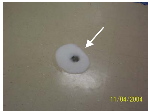
Figure 6. Soap bubbles exiting floor drain during washing machine operation.
