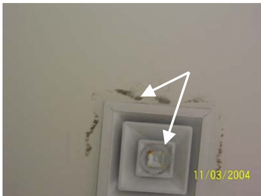
Figure 3. Rust and visible mold on bathroom air supply vent
