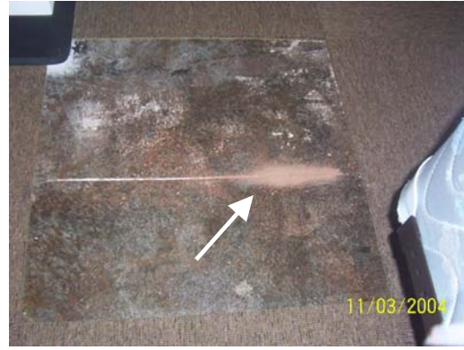
Figure 8. Concrete slab sub-floor with carpet tiles removed. Sand accumulation in the stress control joint.
