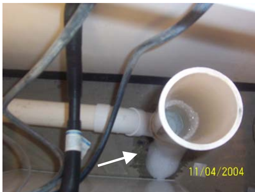
Figure 5. Washing machine sewer drain open to the laundry room. Soap bubbles and water leaking from joints and running onto floor.
