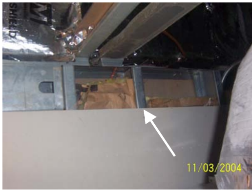
Figure 9. Exterior wall at roof viewed from inside the building above the drop ceiling. Insulation is not continuous to roof.
