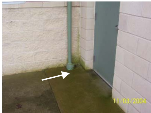
Figure 12. Roof downspout with evidence of puddling and moisture accumulation.
