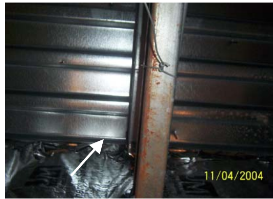
Figure 10. Station 21 - Underside of roof. Roof support with visible rust.
