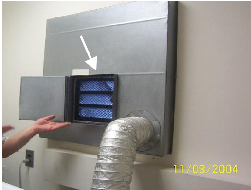
Figure 7. Dryer exhaust configuration. Dryer exhausts into metal box, exits at filter (arrow).
