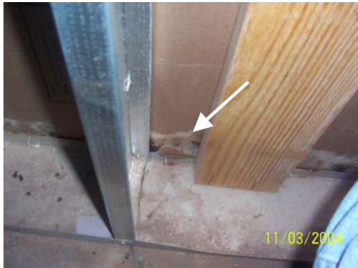
Figure 1. Visible mold and water damage in wall cavity (plumbing chase)
