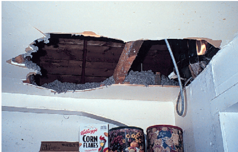
Appendix F – Picture 2. Safety concern – hole created from employee falling through ceiling during preparation of attic for future CI application.
