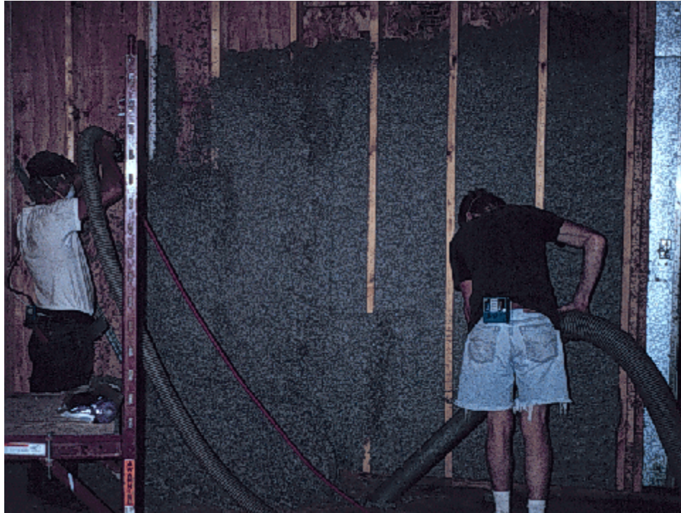
Appendix F – Picture 5. Example of a wall-spray CI application and the vacuum for recycling of excess CI directly into large hopper.
