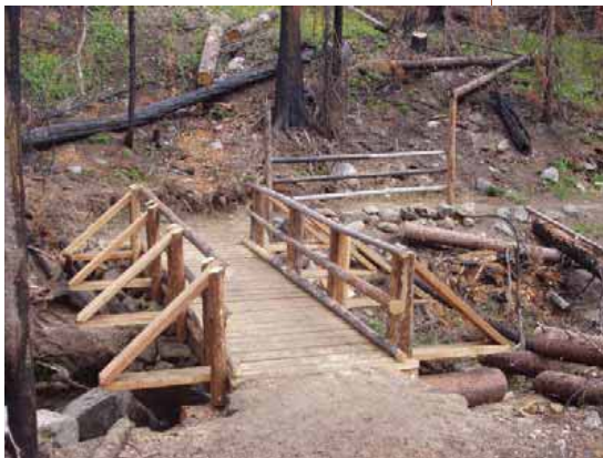
The Peak Creek bridge was reconstructed thanks to the combined efforts of the SKY volunteers, Backcountry Horsemen and Forest Service Employees. The bridge had been burned during the 2003 Isabel fire.
