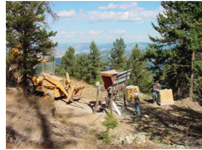
The exploration bore holes must be plugged with bentonite 50’ above the static water level, then sand can be used to within 25’ of the ground surface. This is to insure there is no water aquifer contamination with surface water. The project plugged over 750 bore holes in 2002.
