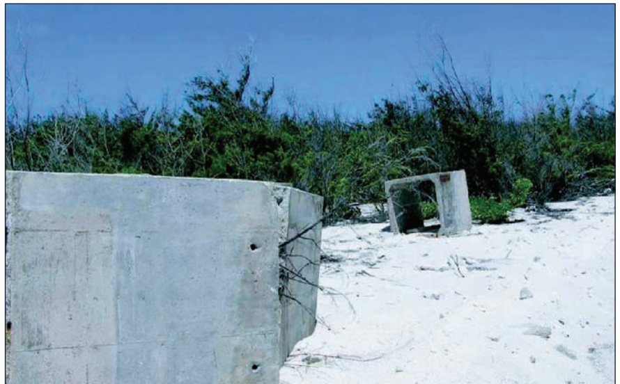
Figure 11.11 Concrete blocks filled with sand and coral rubble to form a seawall were carried tens of meters up the beach on Wake Island. Photo: J. Miller.
